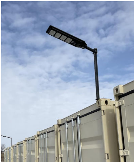
IN USE — SOLAR AREA-LIGHT MAST
