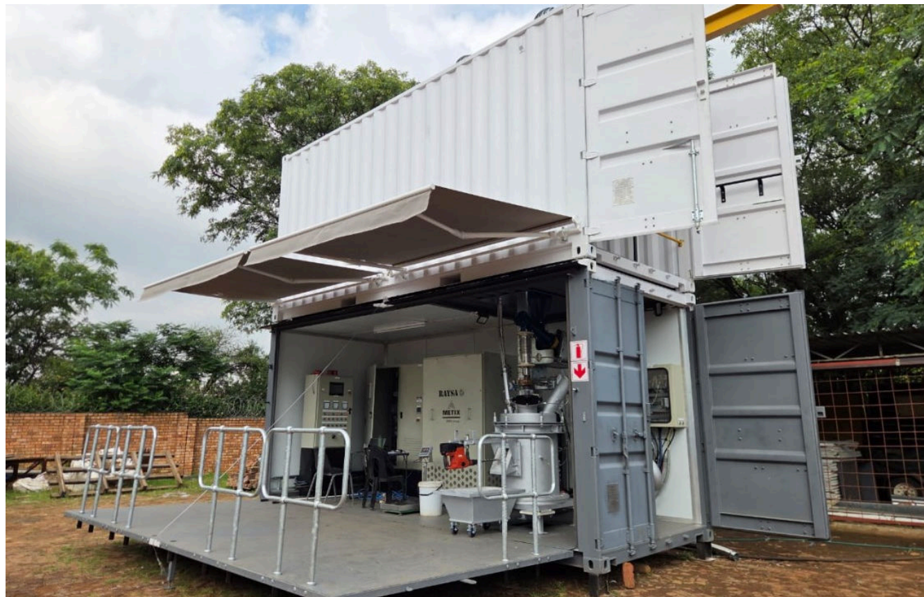
THE CONTAINERISED H 2 TEST FURNACE INSTALLATION AT POTCHEFSTROOM UNIVERSITY
